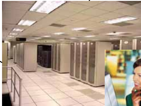
IVECO Back-end Infrastructure
